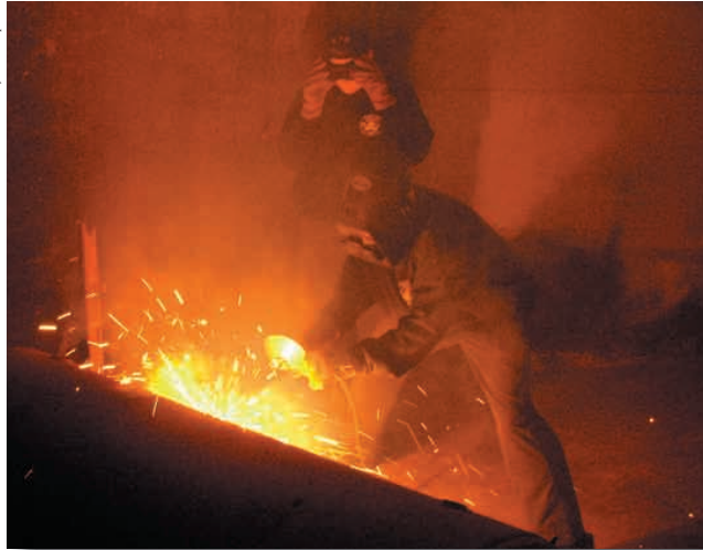
With Safety Signal gone, volunteers were able to help cut up two huge expansion tanks. The original heating system was hot water and when it was converted to steam, these tanks were left in the basement along with many other obsolete pieces of equipment.
