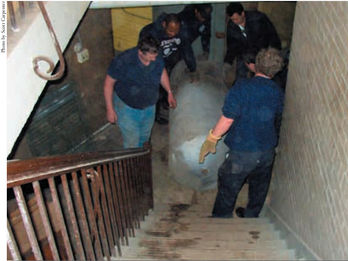
After cutting up the expansion tanks, Firefighter volunteers help haul them out of the Museum basement.
