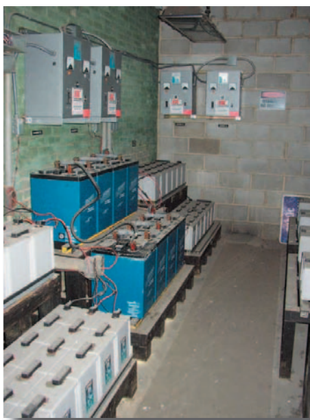
Even before Safety Signal vacated the building, volunteers removed 150+ batteries from this room.
