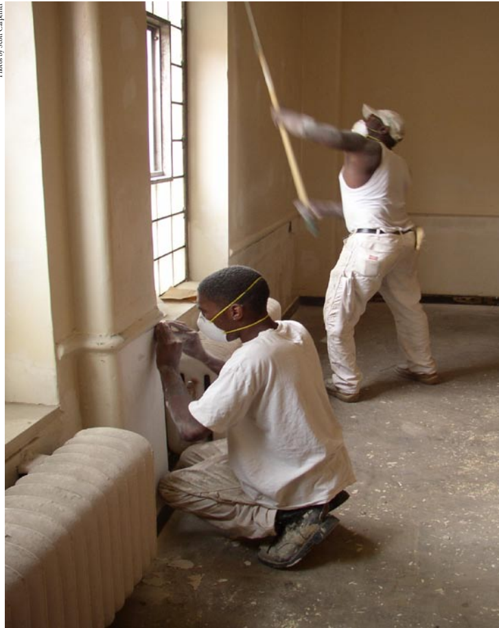
Post Painting came to the rescue in August. Louise Post sent four of her best painters to help out. Here are two of them hard at work in the Day Room patching, sanding and priming the walls and ceiling. Volunteers will be finishing the job in the very near future.
