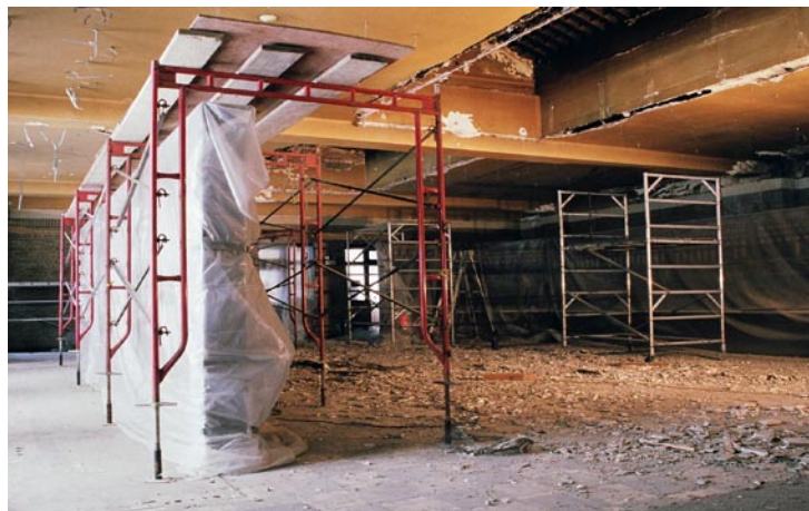
Over the last couple months volunteers have made great progress. Much of that progress was in the Alarm Office and Dispatch. Walls and ceilings have been completely removed. The week after this photo was taken, volunteers began removing whole sections of the badly damaged ceiling and as of October 1 st that work is done.
