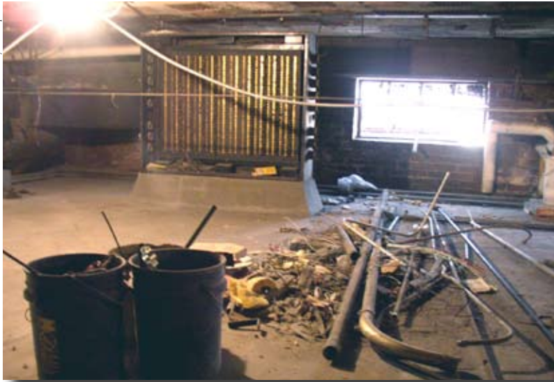
Volunteers Paul Bobak, Jim Hart, Ray Ross, Bill and Mark Storch, Stuart Warner and Project Manager Scott Carpenter toiled for more than a month of Thursdays in the four and a half foot high crawl space known as the Mezzanine, cleaning out old wiring, buckets full of debris and much more. The dumpster was filled every two weeks and Mark Storch took several loads of scrap metal to the scrap yard raising hundreds of dollars for lunch and other expenses.
