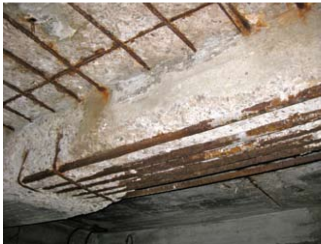
These photos were taken of the underside of the apparatus bay floor.
