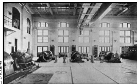
Operating Room of Pumping Station
